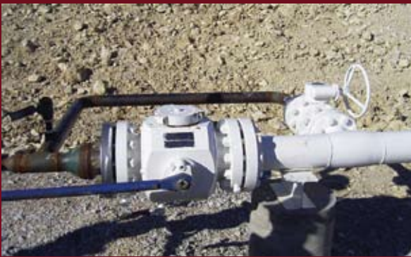
Barnett Shale, 6" 600 ANSI Launching valve, with reduced bypass.
